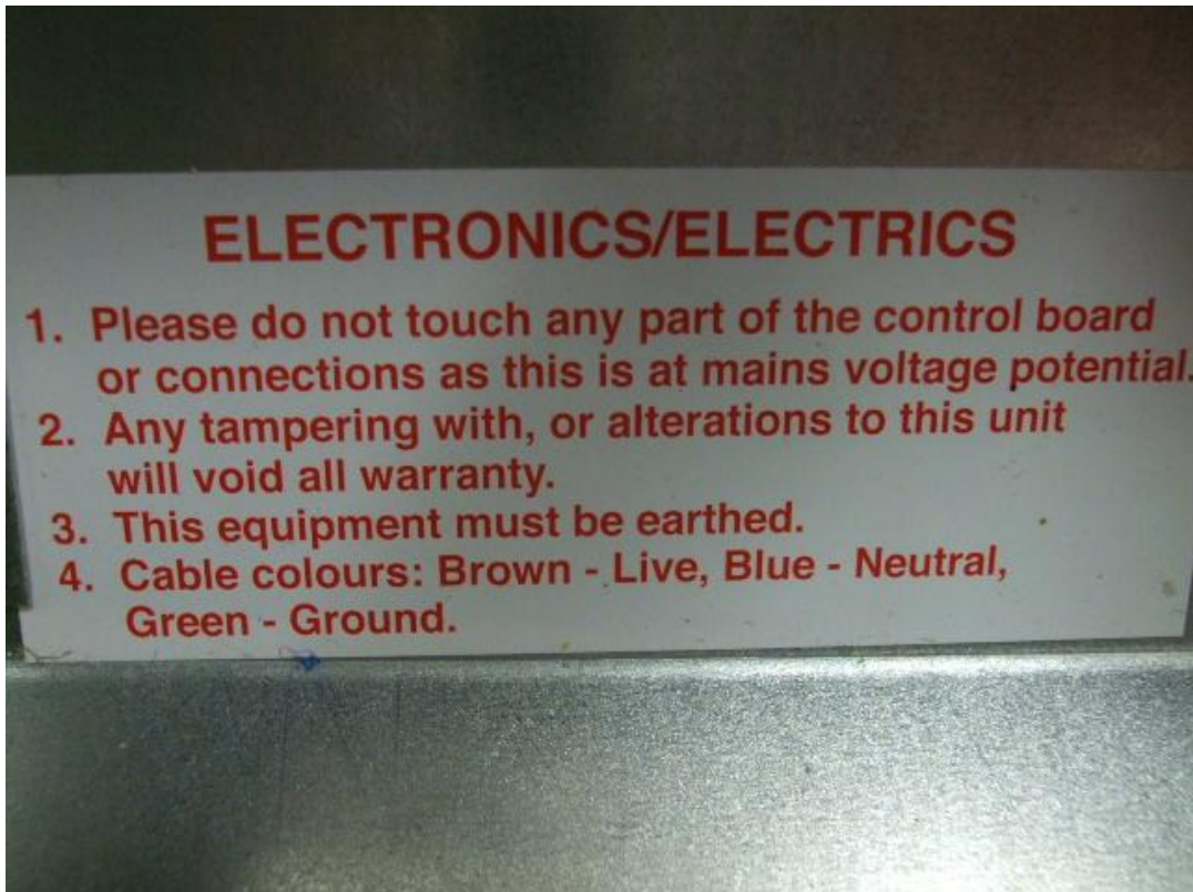
Electrical installation safety labeld
